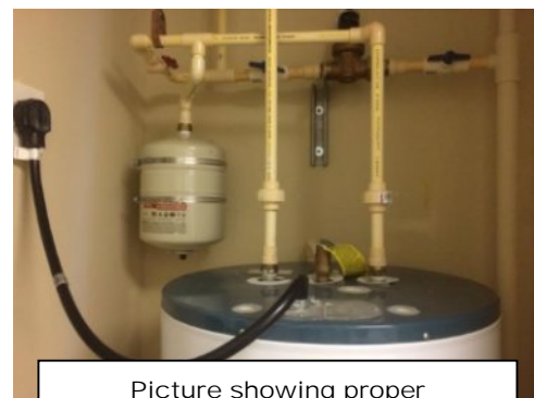
Picture showing proper installation of expansion tank and pipe supports.
